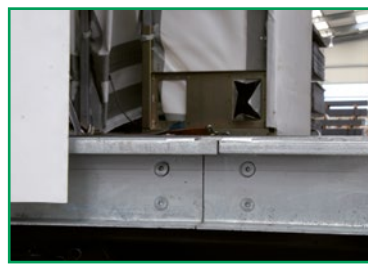
Laufschiene aus Stahl in Segmenten verschraubt Running rail made of steel, bolted in segments
